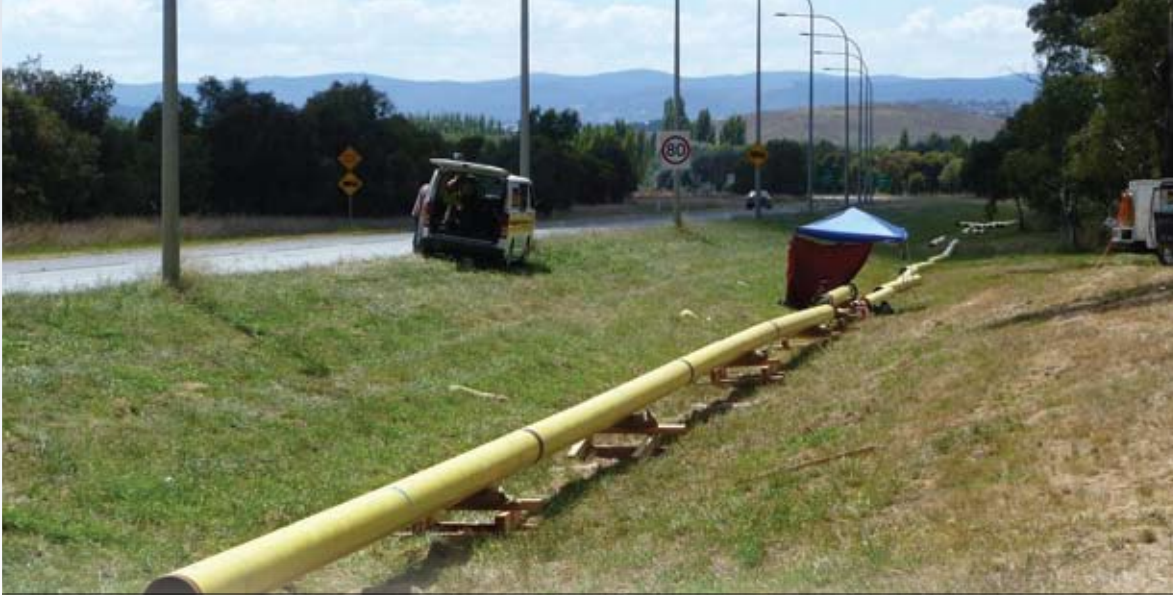
Stage One of the Hume to Tuggeranong interconnection project was completed during the year. The project will support future growth in these areas and ensure continued supply over the next 20 years.
