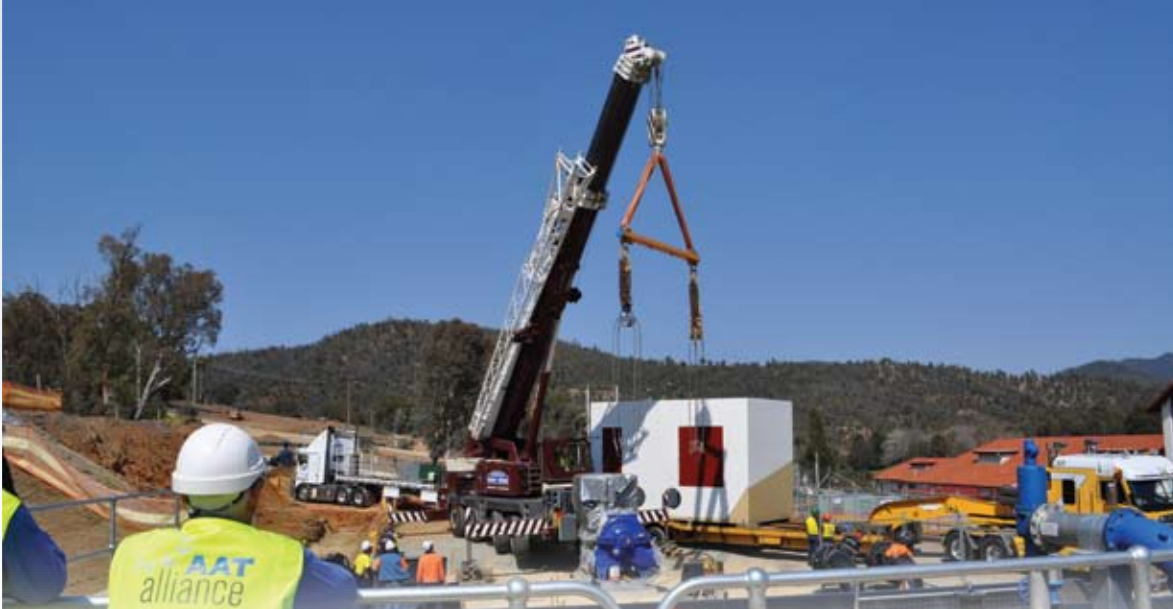
The AAT alliance successfully commissioned Cotter Pump 10 during the year.
